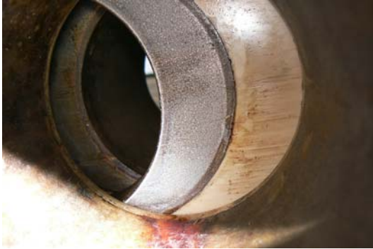
Example of metallic scale formation. Valve in service in partial open position
